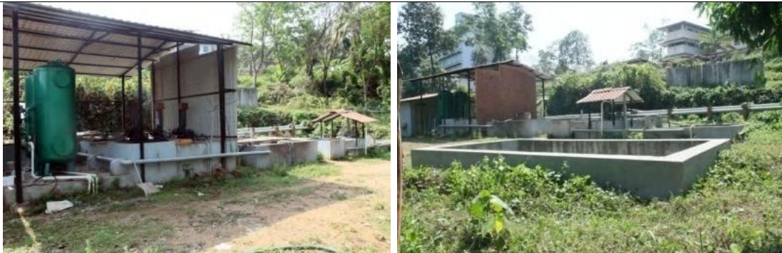
Waste Water Treatment plant – 2 lakh capacity
