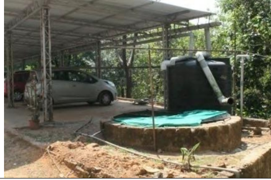
Rain Water Harvesting - Recharging the well
