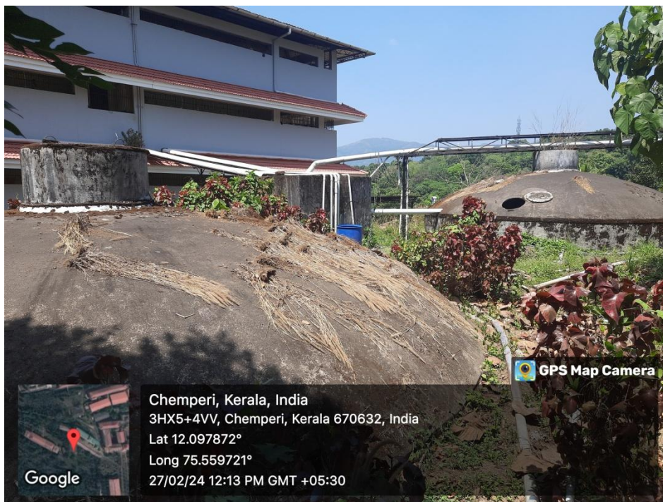
Ground submerged twin Rain Water harvesting tank near Sanjose Boy's hostel
