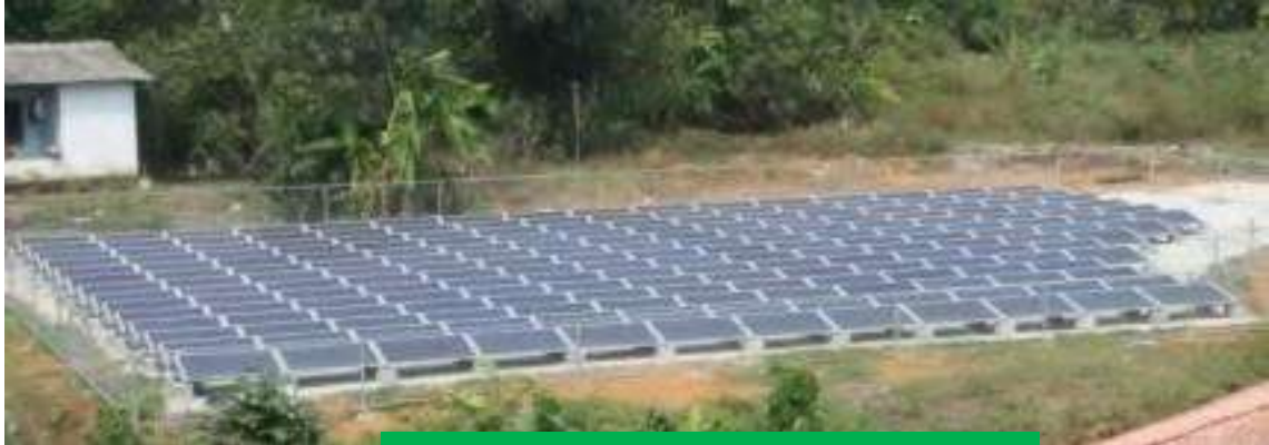
50 kW Solar Field – Various Views
