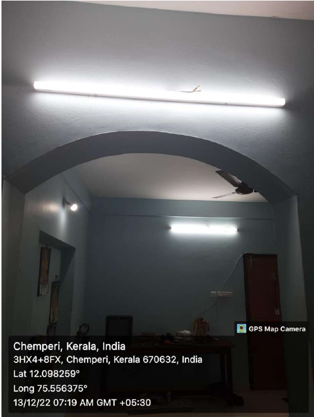
LED Tube Light and LED Bulb in Staff Quarters
