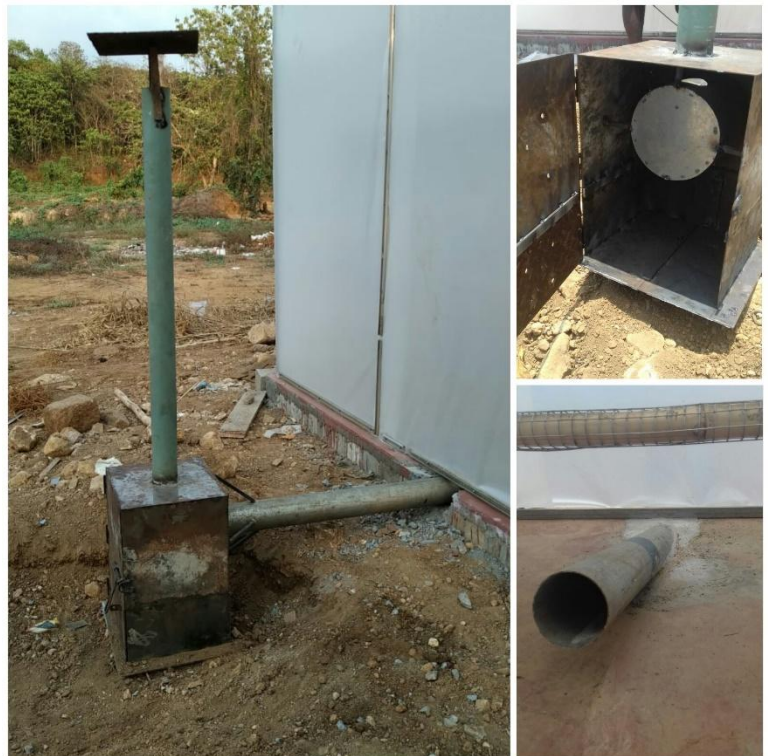
Figure 6: Biomass backup heater
