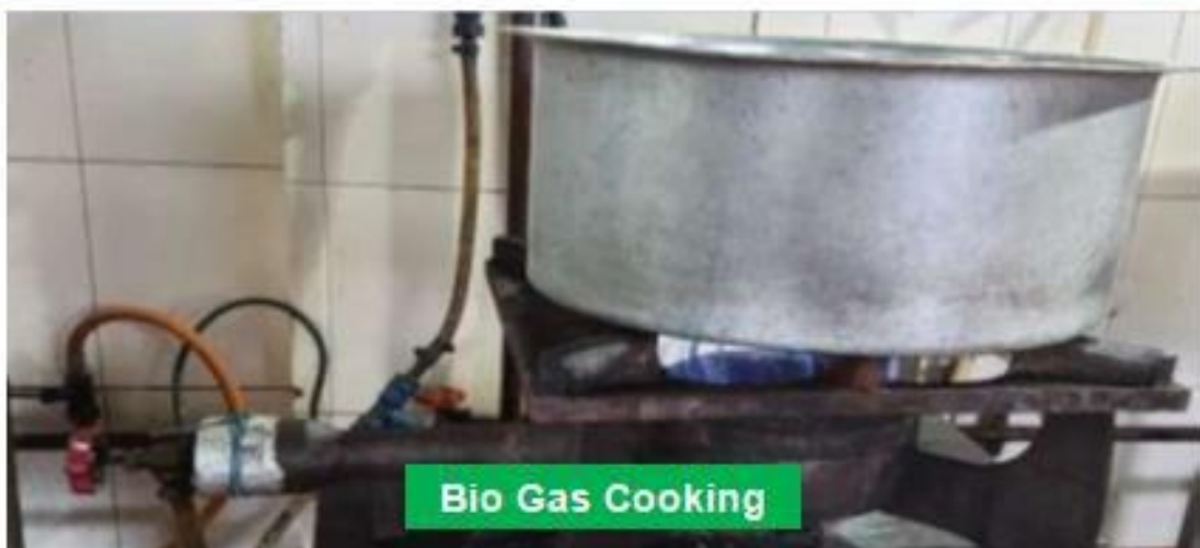
Bio Gas Stove and units
