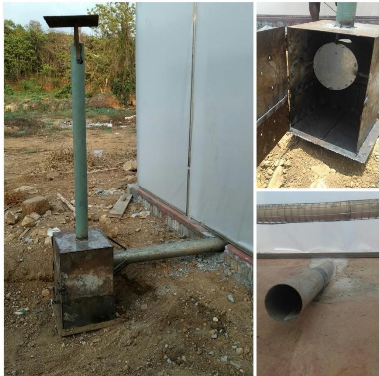
Figure 6: Biomass backup heater
