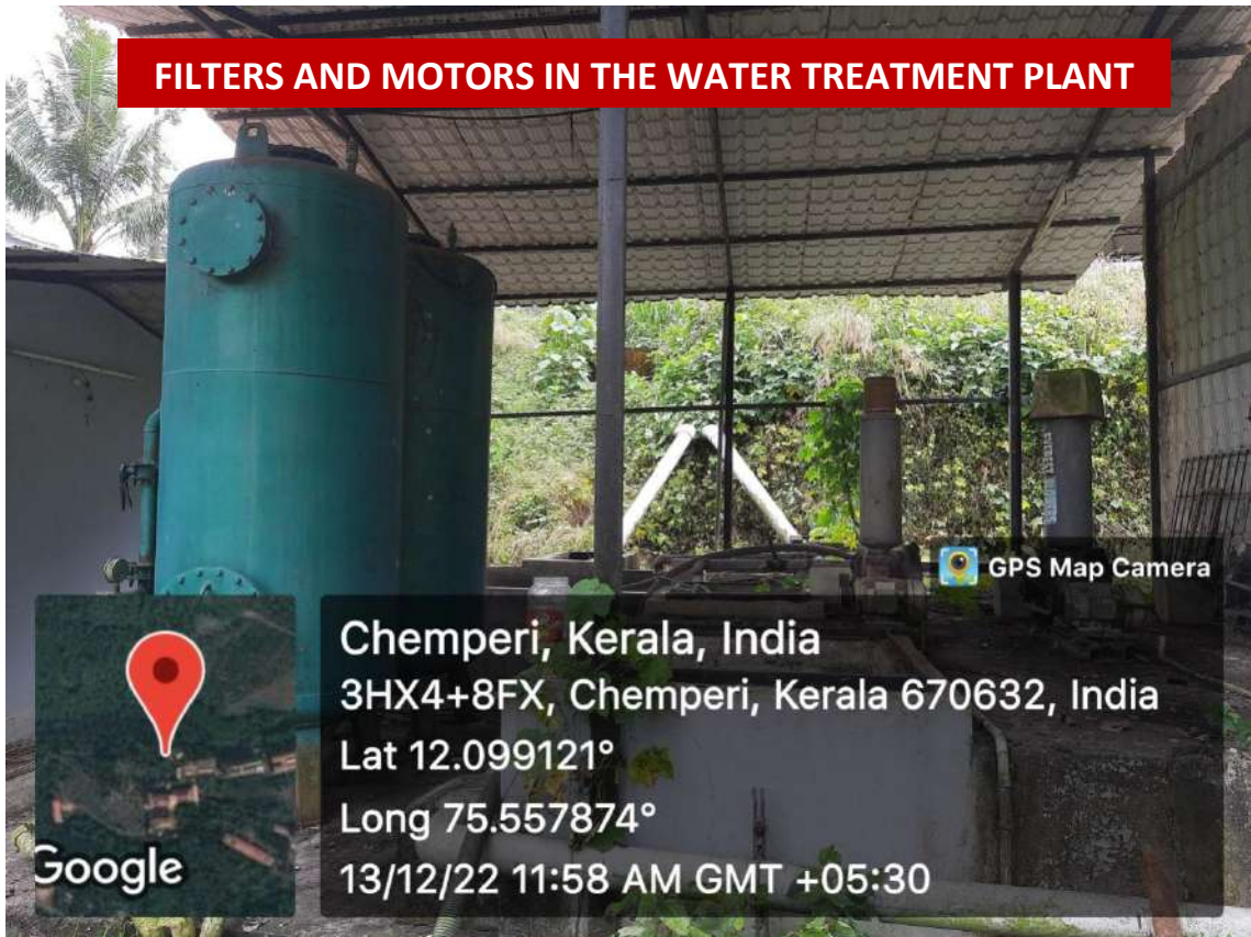
OVERVIEW OF THE WASTE WATER TREATMENT PLANT
