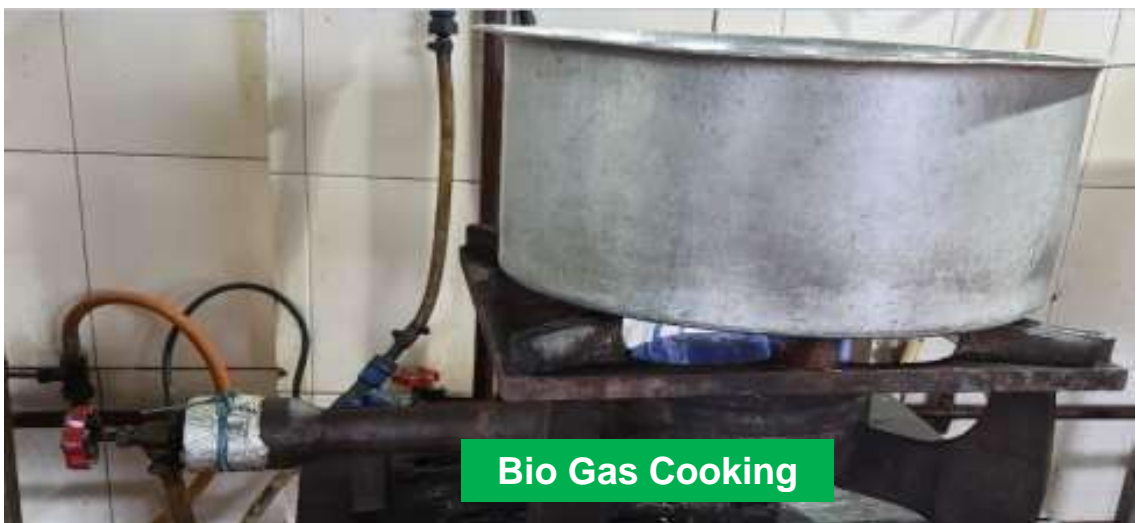
Bio Gas Stove and units
