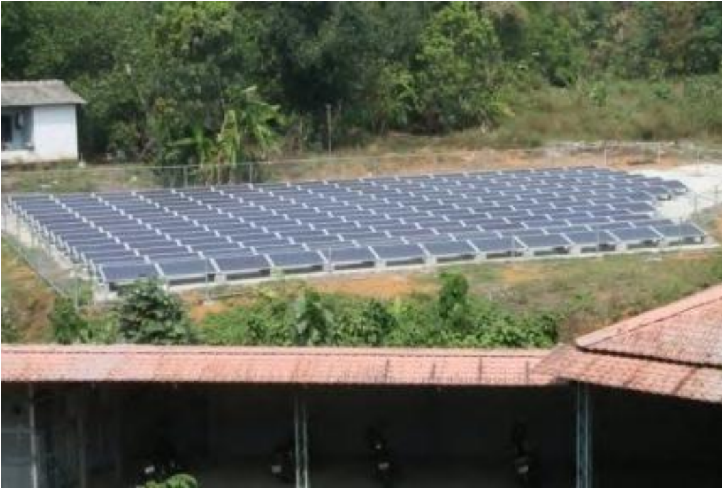
Solar panels on ground
