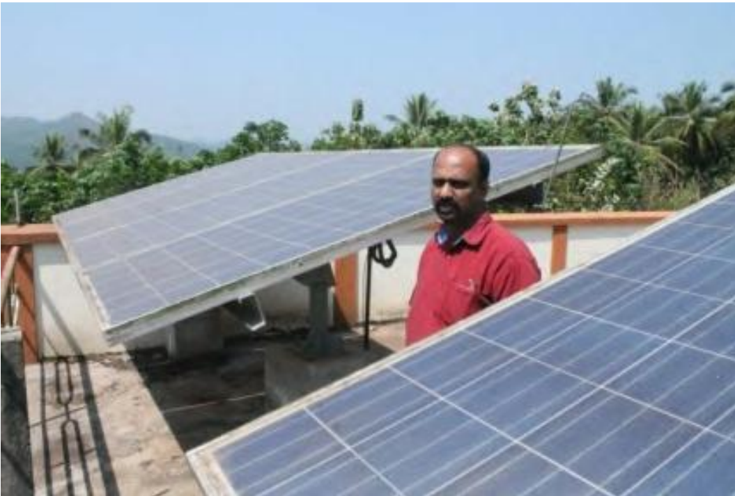
Solar panels on Roof Top
