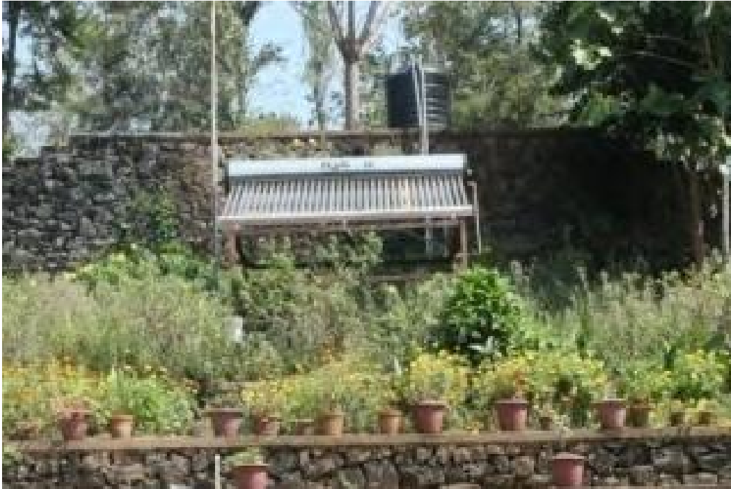
Solar water Heater
