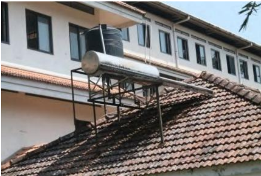
Roof top solar water heater
