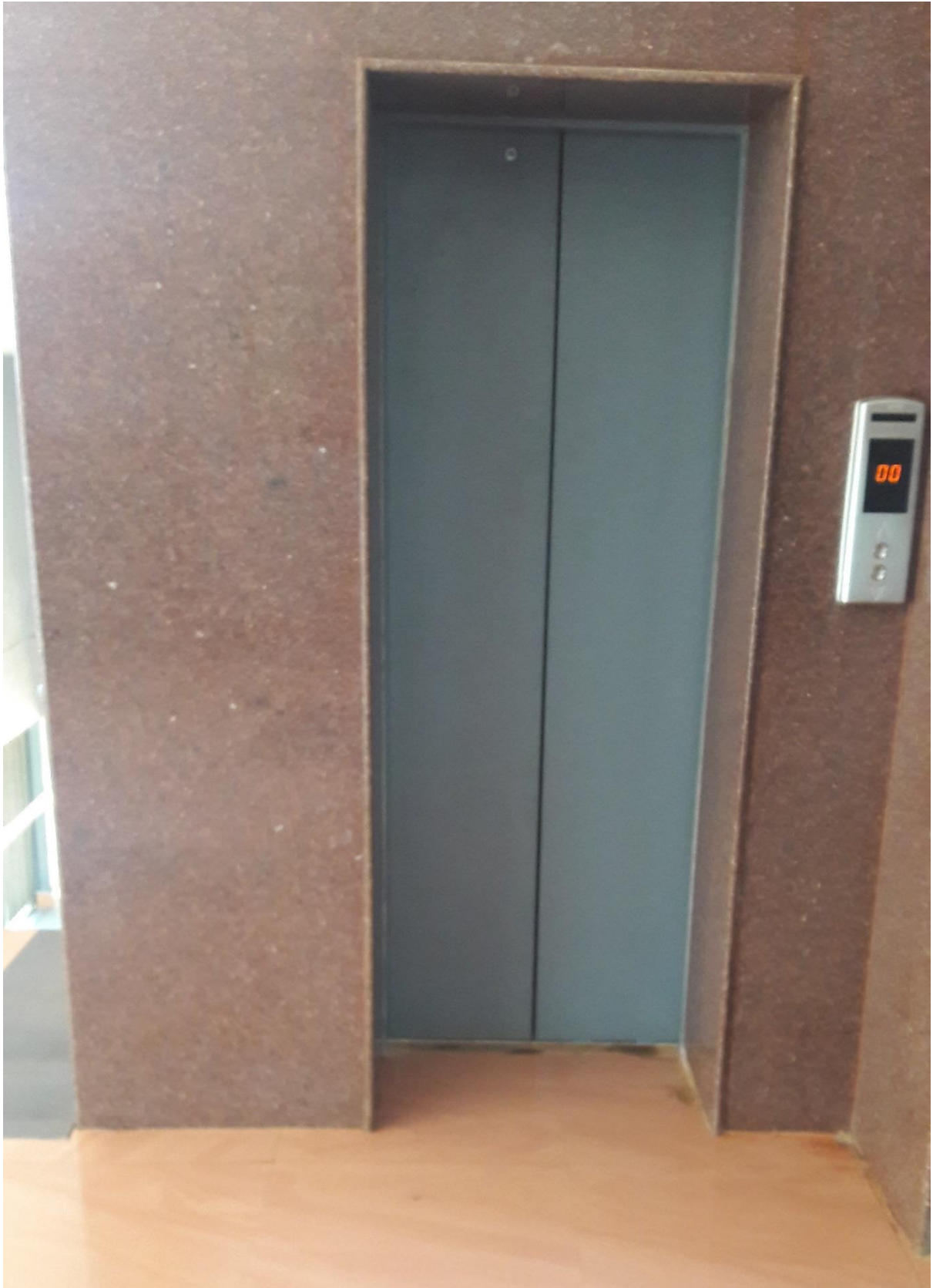
Operational lift – Idle at Ground Floor
